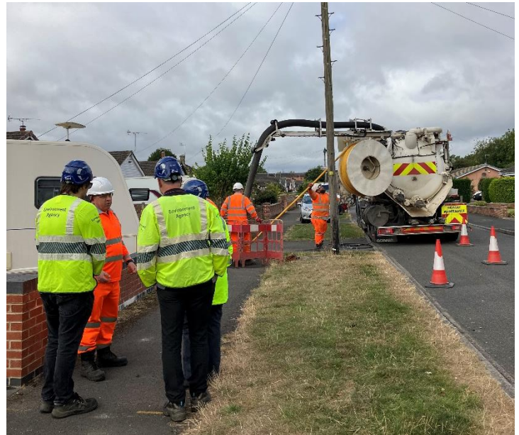
Figure above: EA staff speaking to AMCO Giffen about the culvert de-silts
